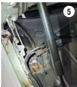
5 THE ROOT CAUSE of many interior water leaks is clogged drains.
