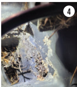
4 DEBRIS PRESENT makes a clogged sunroof drain a likely suspect.
