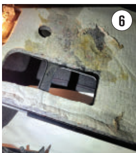
6 EVIDENCE OF WATER ingress is present.
