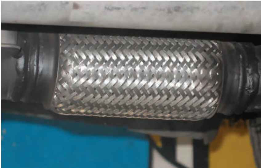
Common sources of air leaks into the exhaust system that can skew the ECM's tests include damaged flex pipes and stripped or damaged sensor threads.
