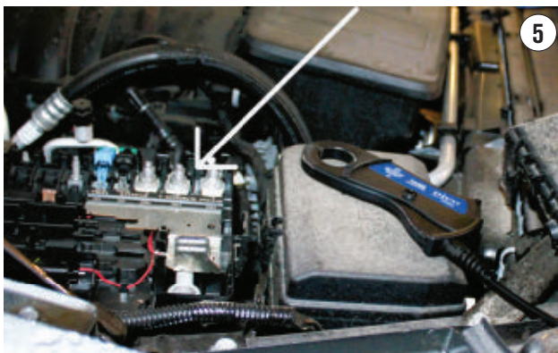
POSITIVE BATTERY CABLE terminal fusible plate.
